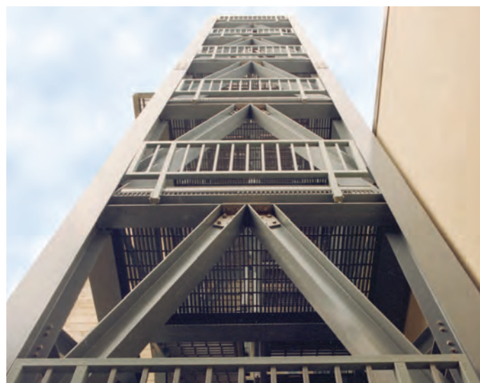
A 63' (19.2m) high freestanding fiberglass stair tower at Ft. Story Army Base, Virginia Beach, Virginia.
