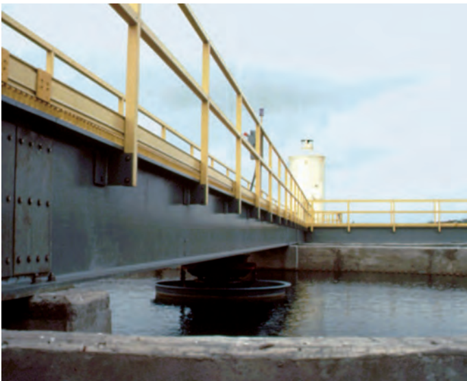
Lightweight, corrosion resistant 24" (610mm) I-beams span 45' (13.7m) to bridge clarifiers at the Las Rusias, Texas wastewater treatment plant.
