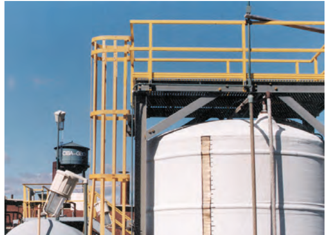
This fiberglass ladder and cage provide worker access to a maintenance platform at a Ciba Geigy plant in the northeastern United States.
